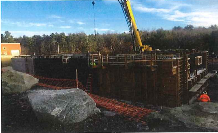
Figure 2 Load Platform for Aeration Basins
